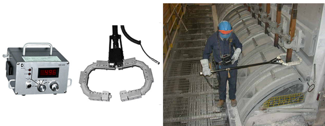
Figure 2.2. DynAmp clamp-on portable (COP) current meter.
